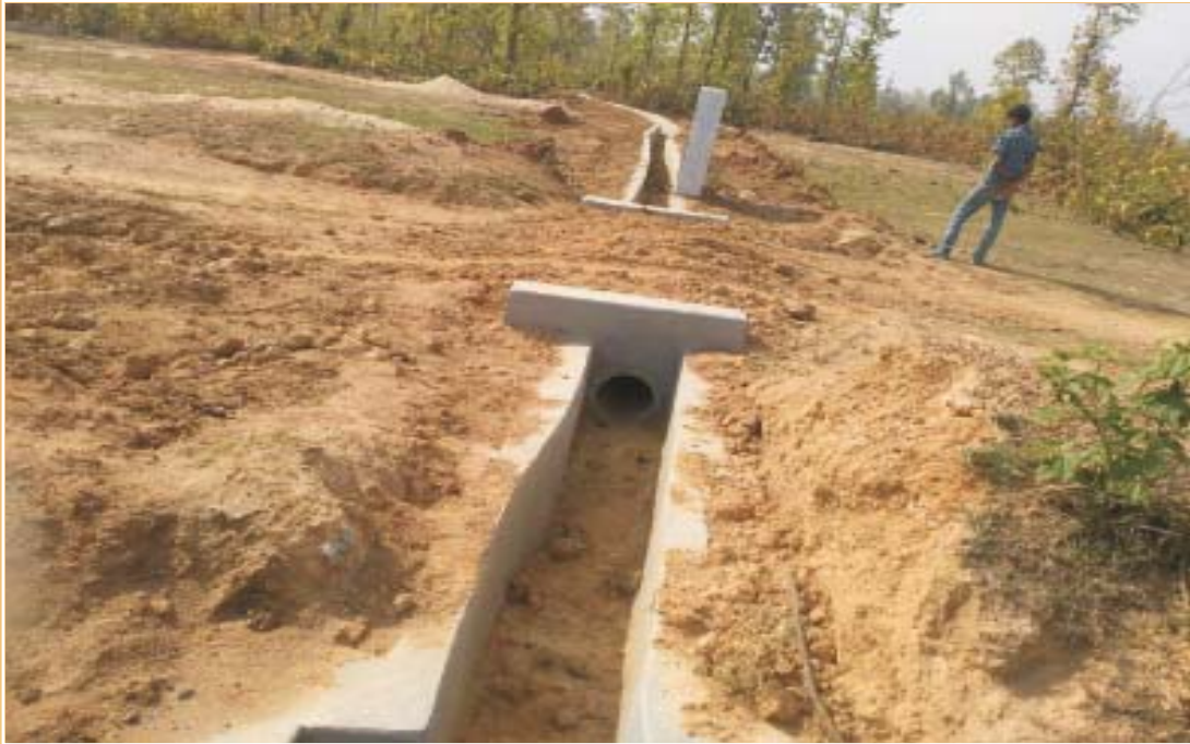
Construction of Field channel scheme at mouza- Patharmari, Piasala G.P. under P.S.- Garbeta-II
