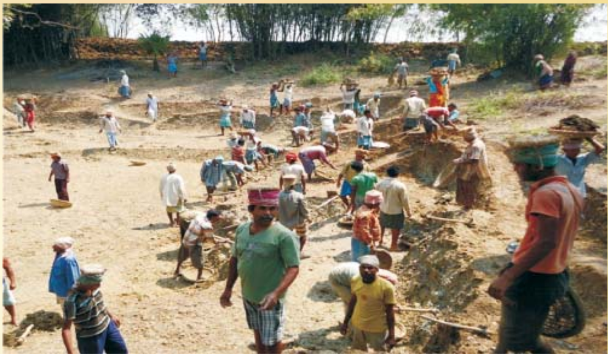
Re excavation of Tank at mouza- Parulia, block- Patashpur, dist- PurbaMedinipur under MNREGA programme
