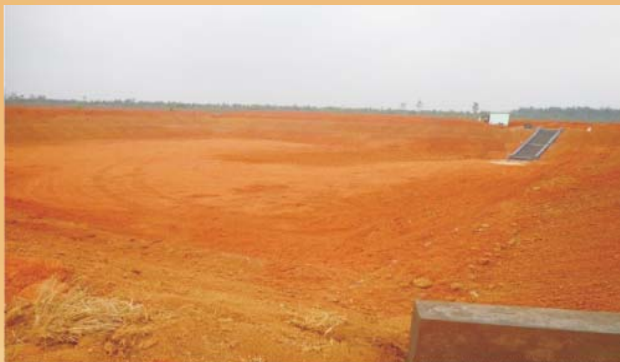
Modernization of Water Harvesting tank at mouza- Marnisole, block- Sankrail, district- Jhargram under Jalatirtha, Phase- II programme
