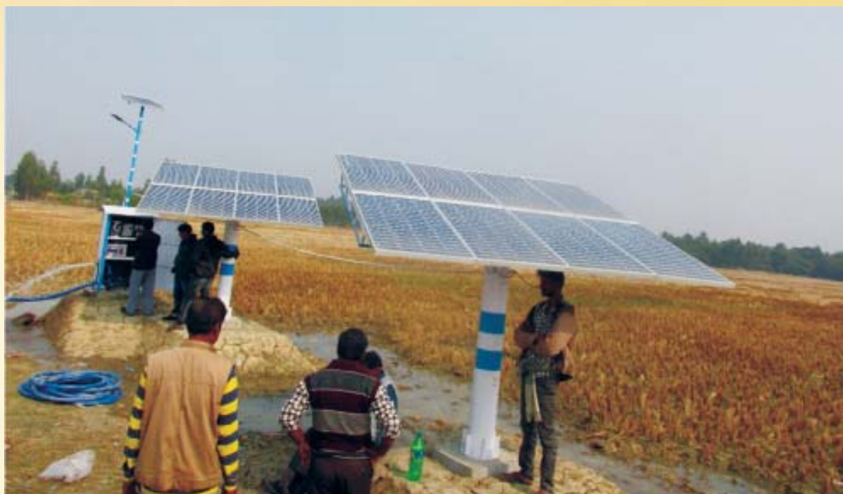
Solar power operated Sprinkler Irrigation system at mouza- Bali, Block - Gosaba, District - South 24 Parganas under RIDF-XXI Programme
