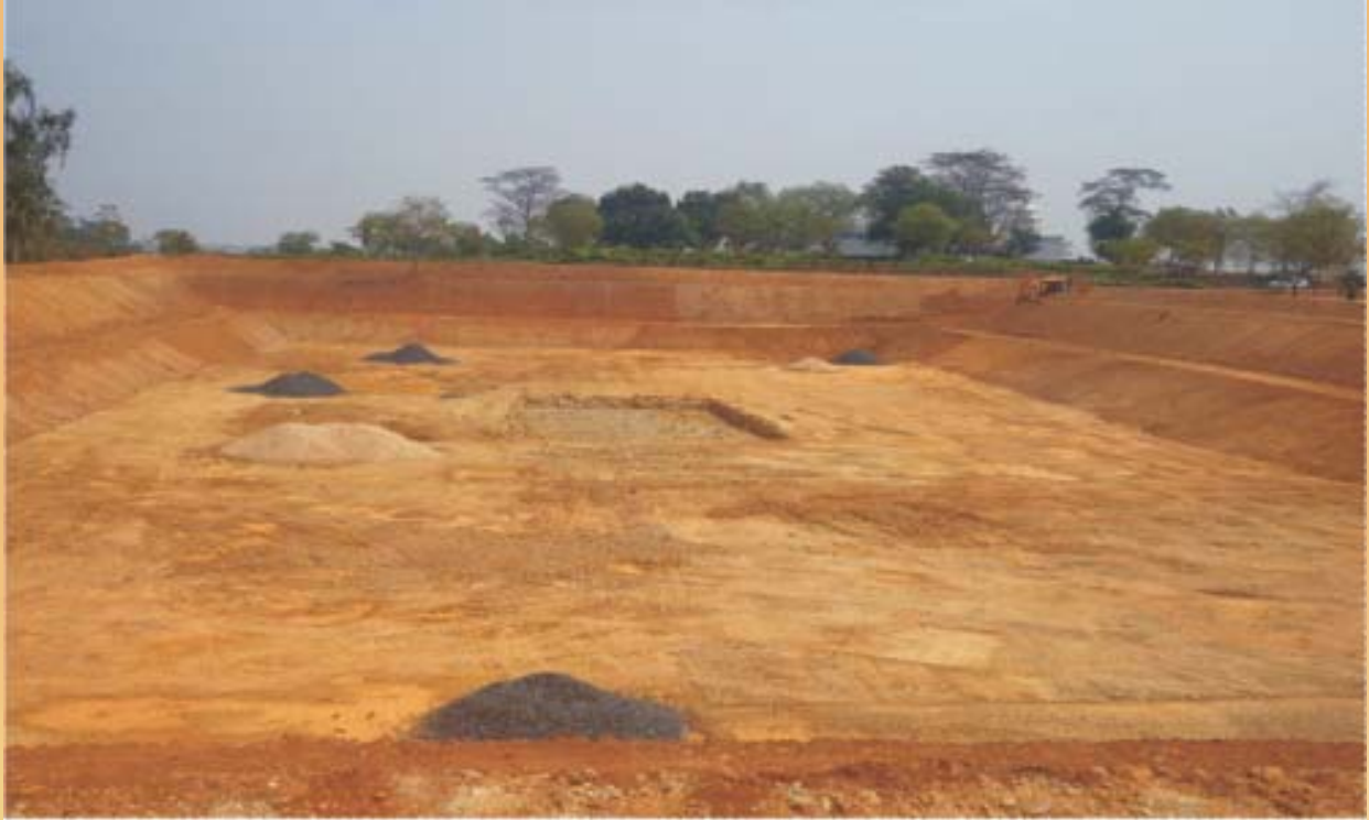
Rainwater Harvesting Tank at mouza- Khatgeria, block- Jamboni under Jhargram district.
