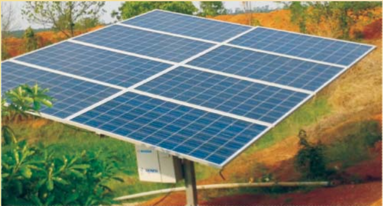
Solar power operated Sprinkler Irrigation system at mouza- Sizdiha, block- Sankrail, district- Jhargram under RIDF- XVIII programme
