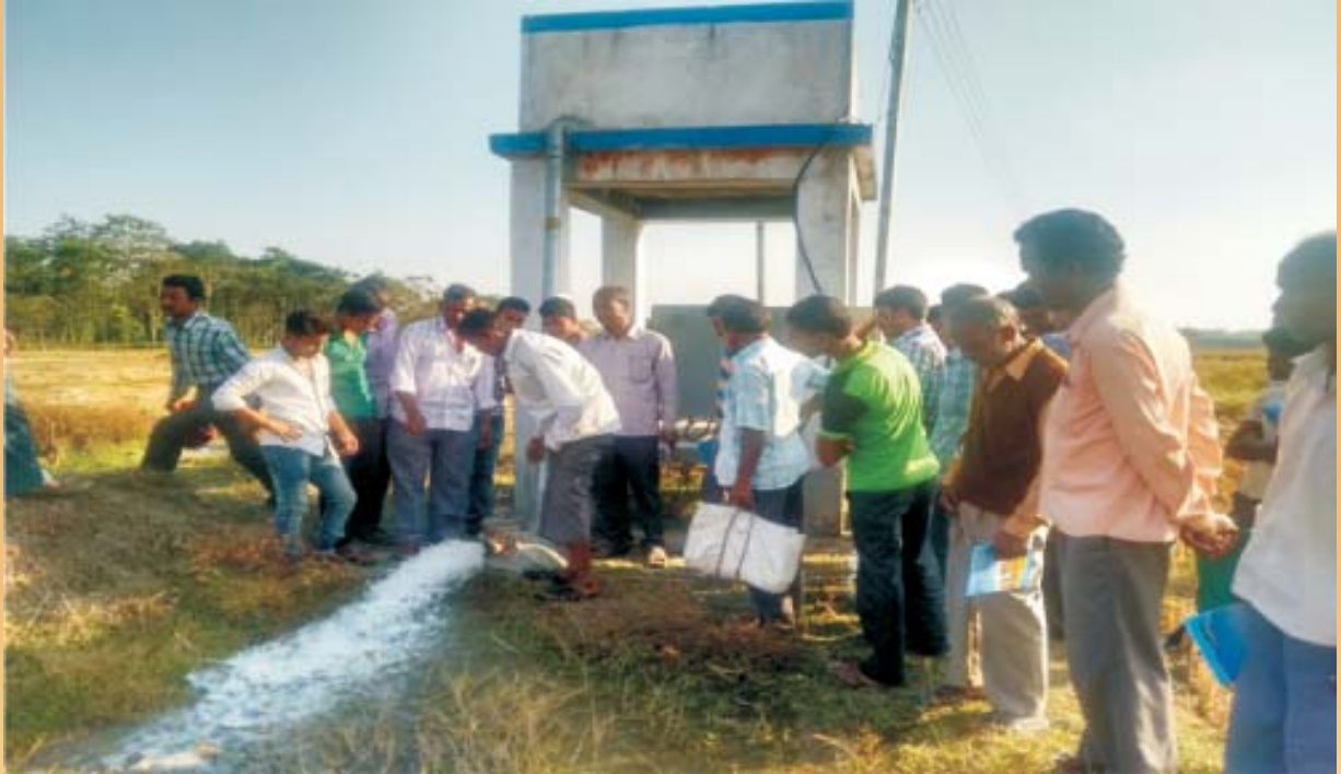
Discharge testing of a scheme before handing over to beneficiaries under WBADMI programme
