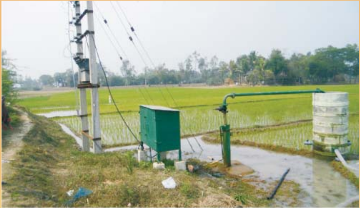
Tube well under WBADMI Programme at mouza- Shaktia, block- Bhagawanpur- II ,dist- PurbaMedinipur
