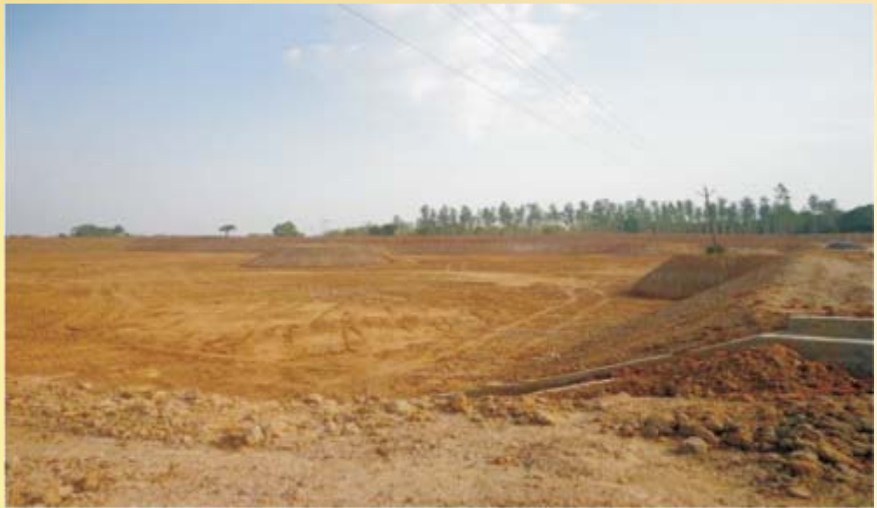
Modernization of Water harvesting tank at mouza- Khasibundh, block- Jamboni, dist- Jhargram under Jalatirtha (phase- II) programme
